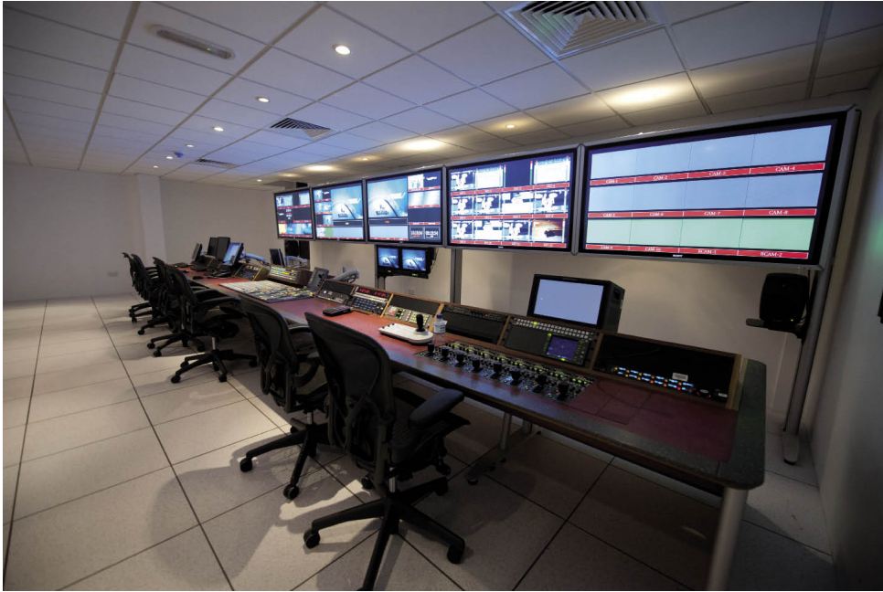
Figure 2.6: A Lund Halsey control room furniture installation
